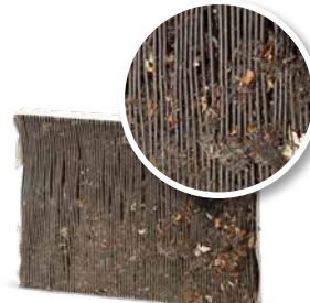
Without A/C maintenance
