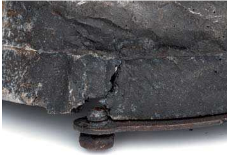
Fig. 1 Crack in the turbine housing
