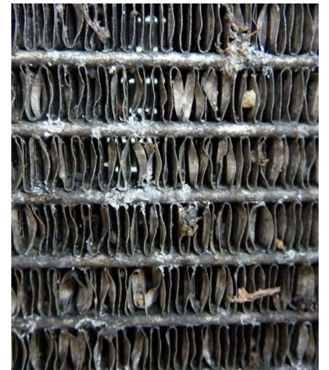
Fig. 2: Contaminants and deformed cooling fins
